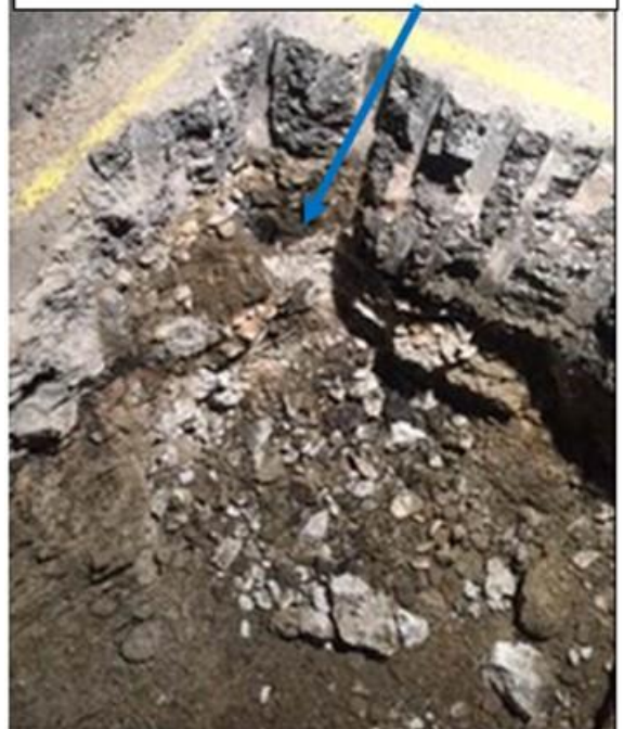
Hole where the hand held heavy air breaker struck the cable
