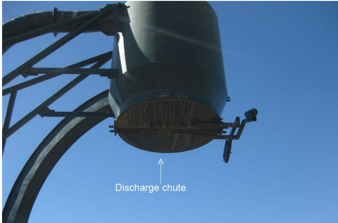
Figure 3: The hopper involved in the incident showing the discharge chute door which failed to seal. Photo by Mine Safety.
