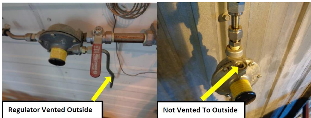
View of Fuel Gas Regulators with and without Venting
